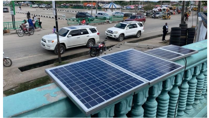
Solar panels from field visit (Photo by Wade Lahring)
